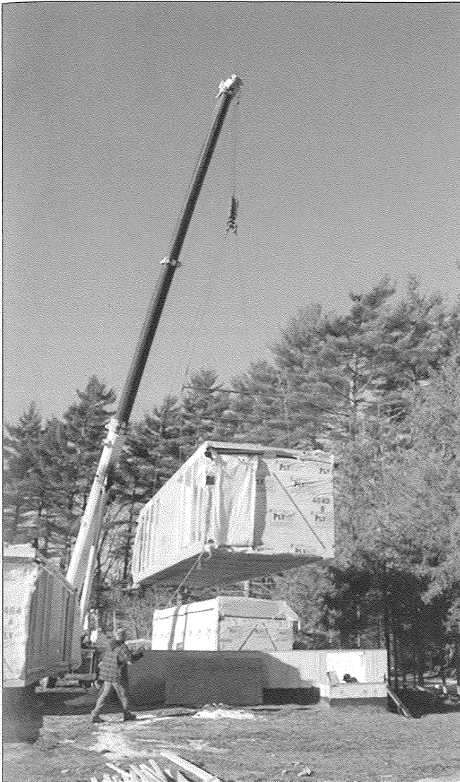
Fig. 2-87. A crane picks the module and mates it to the foundation or the top of another module. Courtesy of Kevin Gallagher.
