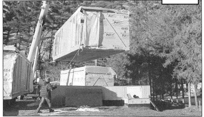
Fig. 2-98. This crane lift point is another easy avenue for fire spread in modular homes. Courtesy of Kevin Gallagher.
