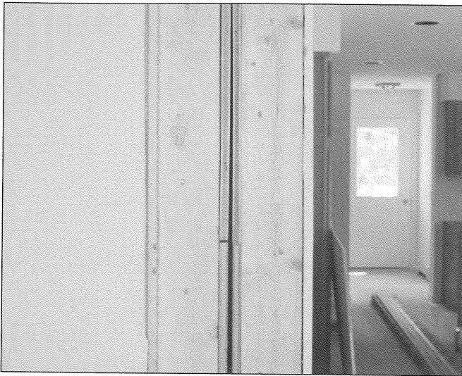
Fig. 2-100. A typical marriage wall between modules with obvious space for fire spread. Courtesy of Kevin Gallagher.
