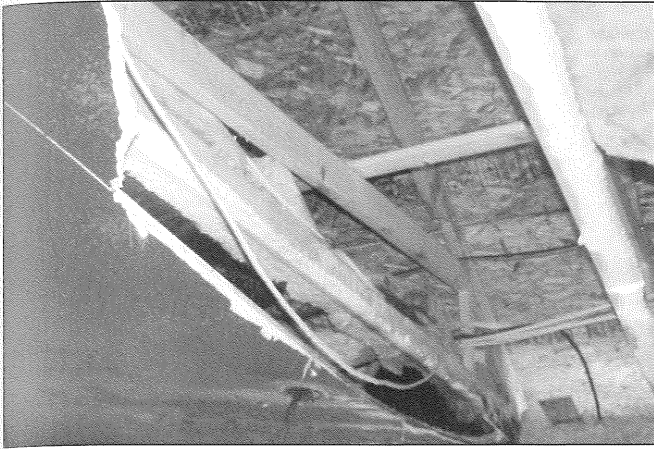
Fig. 2-95. A contents fire has caused the adhesive to begin to fail. Courtesy of Kevin Gallagher.
