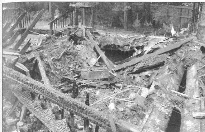
Fig. 2-104. Complete failure of lightweight structural members caused this home to become a death trap for both civilians and firefighters early in the fire. Courtesy of Kevin Gallagher.
