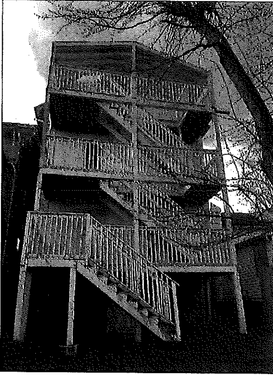
Figure 7-9. Open wood porches present a significant exposure hazard. Courtesy: Matt Kelly
