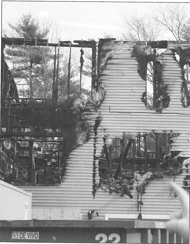
Fig. 2-101. Fire has spread throughout the structure via the void space between the modular units. Courtesy of Kevin Gallagher.
