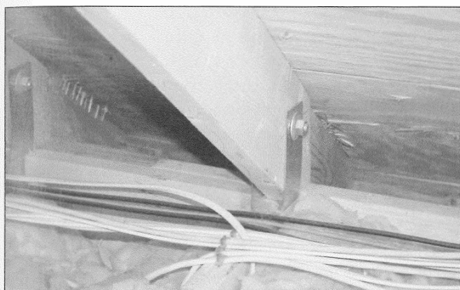
Fig. 2-105. A roof rafter is attached by a mechanical fastener that hinges flat during transport and can swing up at the homesite. This is an obvious structural weak point if attacked by fire.
