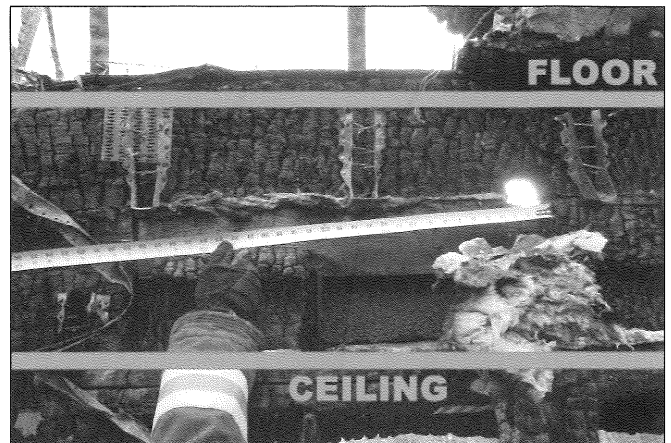
Fig. 2-99. Investigators determined that the lift point helped spread the fire in this case. When properly installed, these holes can be sealed using the materials provided by the manufacturer and the hazard reduced. Courtesy of Kevin Gallagher.
